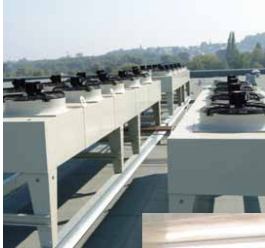
Air conditioning application
